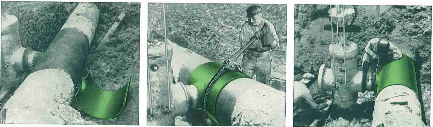
Field photographs showing progressive stages of making branch connection to an in-service line and reinforcing it with the Ladish Split Tee
